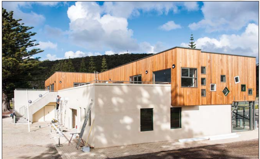
Extensions to the Albany Surf Life Saving Club at Middleton Beach are almost finished.
