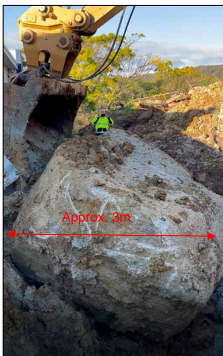
Plate 1: Granite boulder removed from behind 7B Anzac Street
